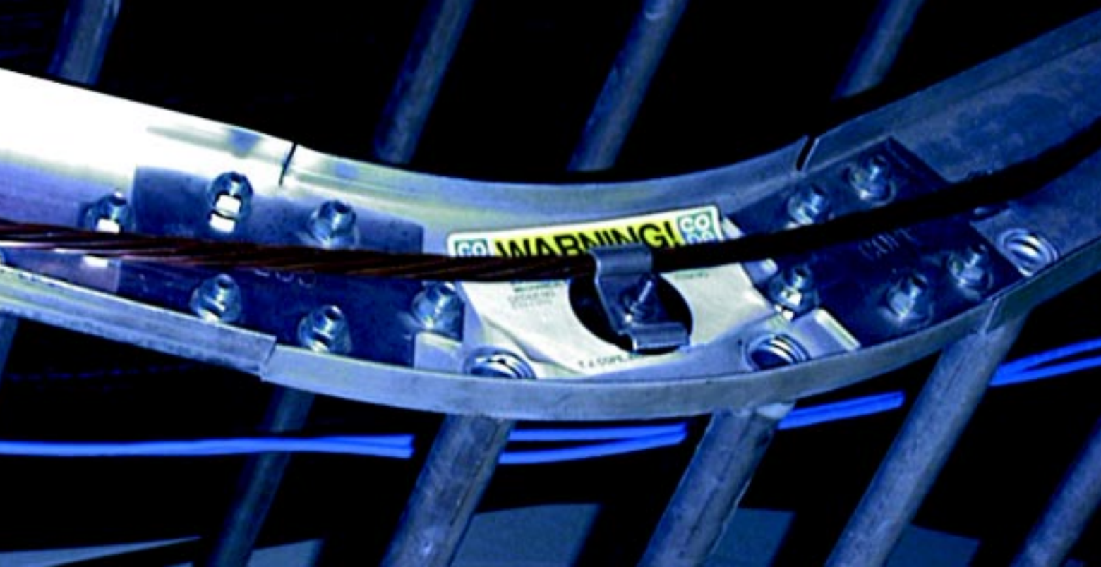
Ladder-type cable tray with external equipment grounding conductor connected.
