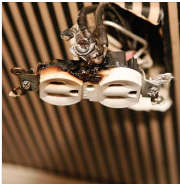
Photo 1. Aluminum wiring incorrectly installed on copper-only receptacle
